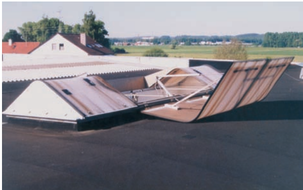
Frameless plastic skylight destroyed by heat and wind, with colouring showing the signs of age.
