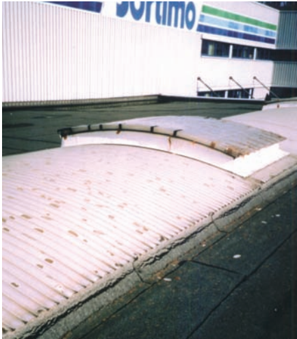
Frameless skylight strip destroyed by hailstones, with single-hipped ventilation flaps.
