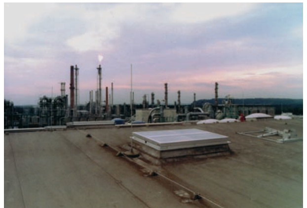
Replaced with Roda Phoenix double-flap ventilator in aluminium section construction with locking mechanism in open and shut state.
