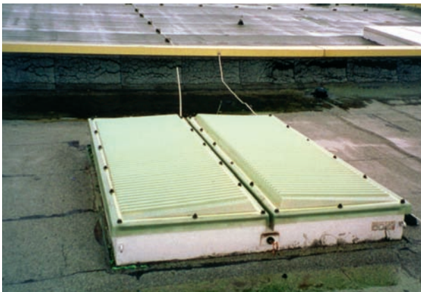
Plastic roof hoods, discoloured through ageing and the effects of the environment.
