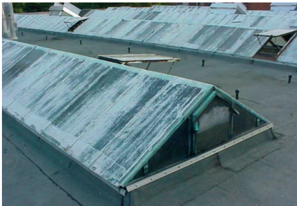
Single-skinned, loose glass skylight, painted with shading paint, with ventilation flaps for fair weather ventilation.
