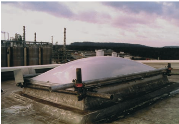
Plastic roof light elements, badly damaged by storms.
